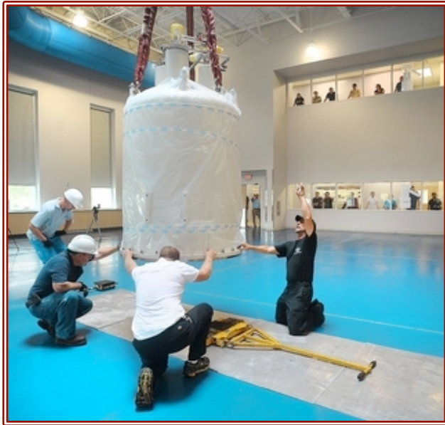
Workers carefully line up placement for the new 800-MHz superconducting magnet which is being installed in the NMR Lab of the Biochemistry Building at TAMU. Eagle photo by Dave McDemand.
